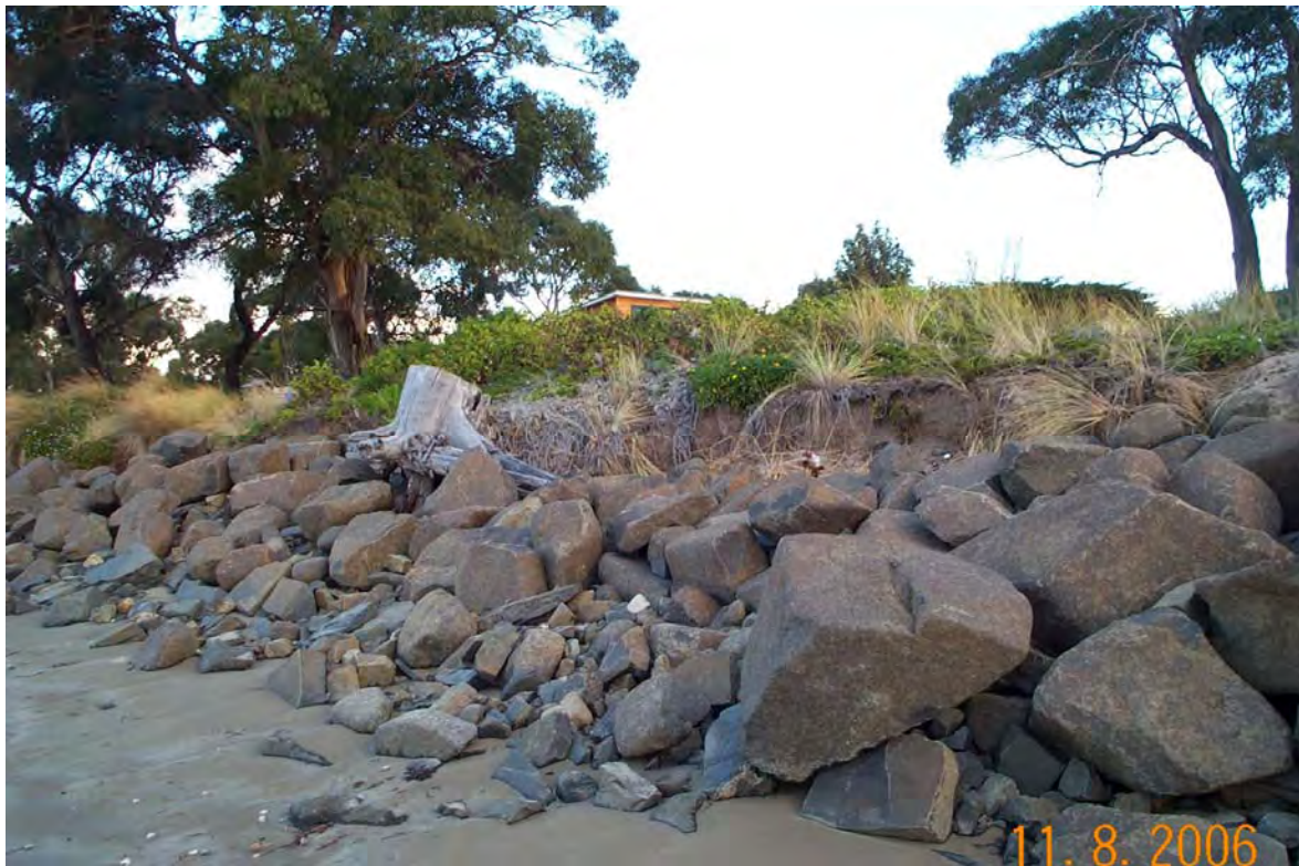
Figure 30: Photo RB2006_26 (Viewpoint 16). This view of the boulder wall (revetment) shows foredune erosion above and behind a section of the wall, indicating that storm waves have begun to overtop and erode behind the boulder wall in this area.
