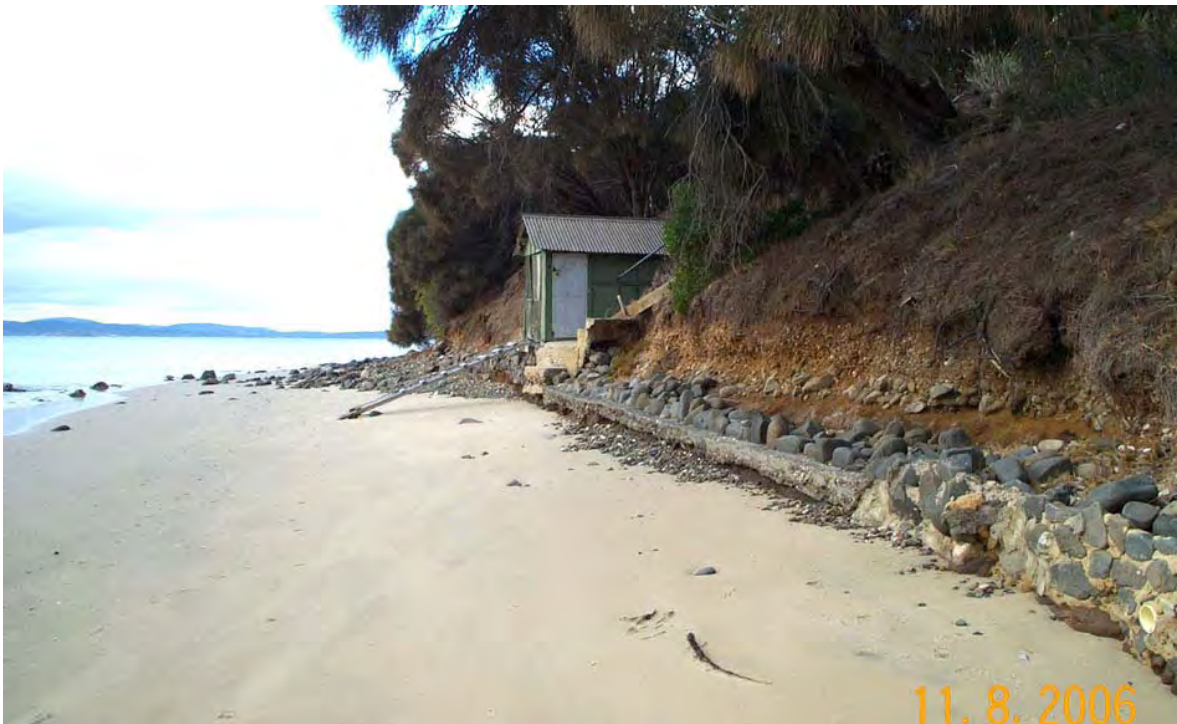
Figure 27: Photo RB2006_6 (Viewpoint 5). An old erosion scarp is evident in places behind this southern part of Roches Beach, eroded into (partly) colluvial soil over weathered bedrock. The artificial wall seen here is evidently ineffective in stopping erosion, however only a small amount of net erosion has occurred here over the last 50 years, insufficient to be detectable as net recession on air photos.
